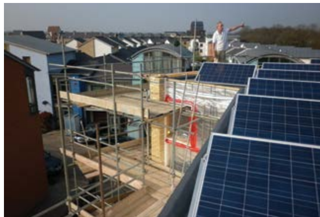
Figure 12.9 Panneaux solaires photovoltaïques
